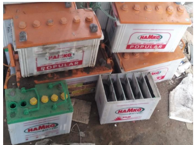
Fig.3: Wasted batteries due to lack of maintenance
